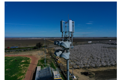
Pierce HS Football Field Light Pole - 4 Radios
